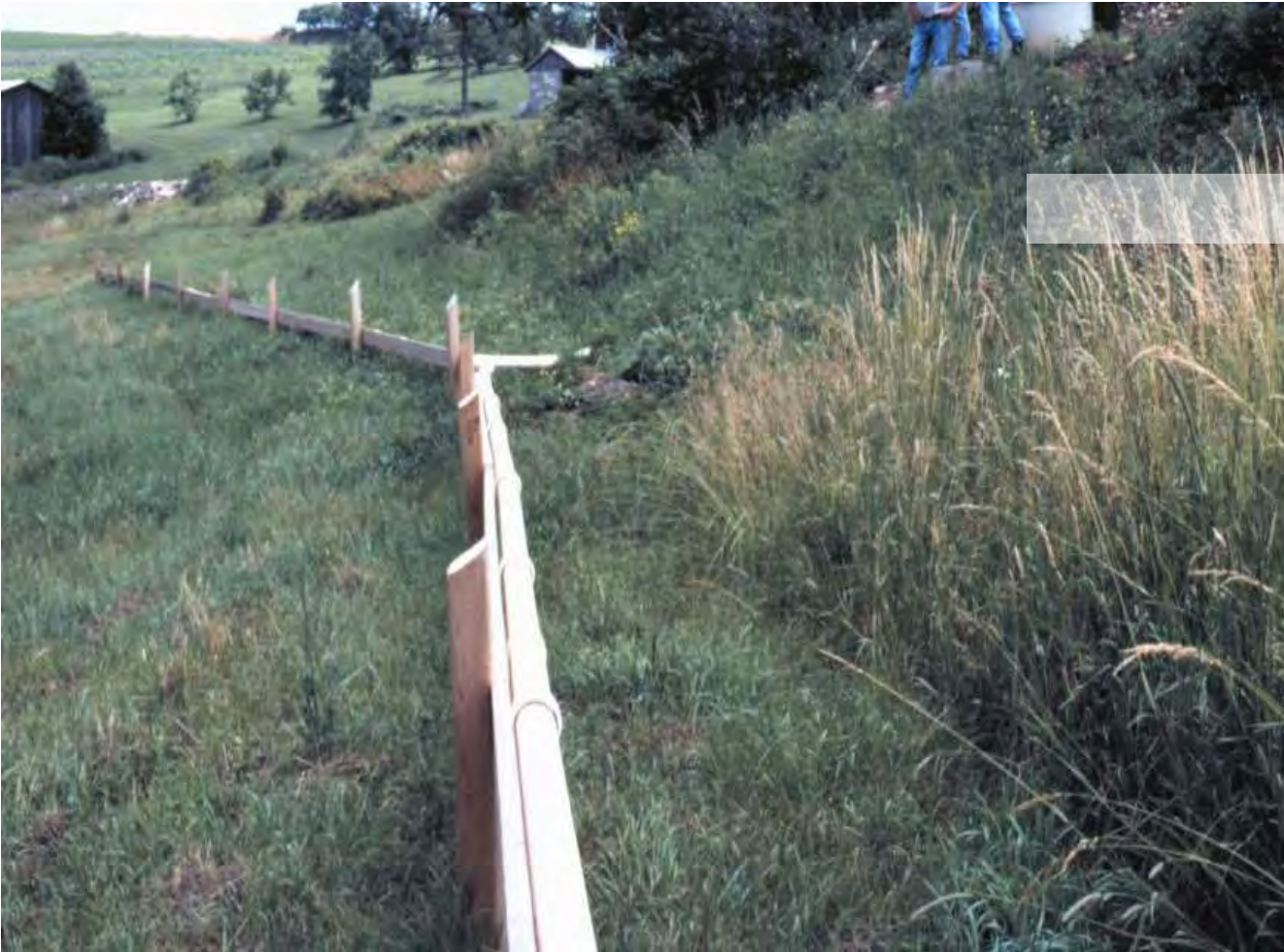
Manure Transfer (634) Gated pipe above a Vegetated Treatment Area
