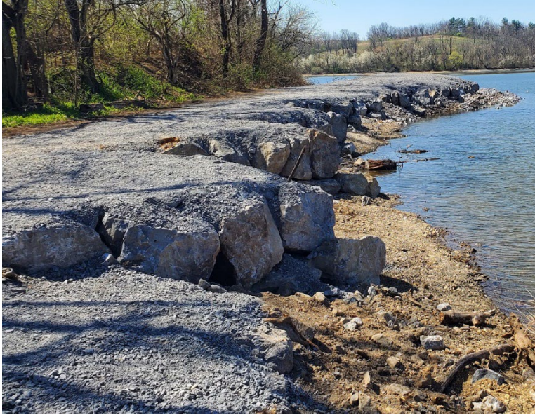
Figure 3-5: Old Church Road Access - Stone Framed Deflectors with an improved kayak and small craft boat slip. The lake is beginning to fill to summer pool elevation.
