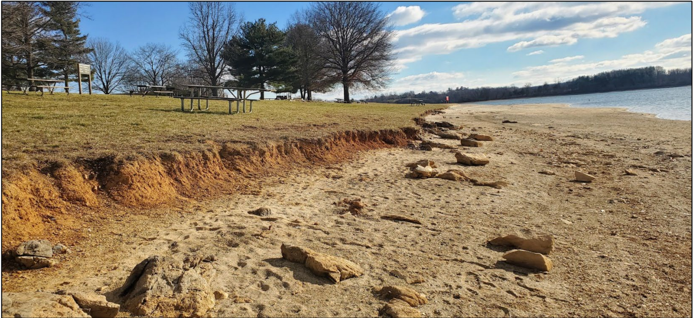
Figure 1: Shoreline erosion from wave and wake action at the Dry Brooks Day Use Area. The area is popular swimming and picnic area and is highly used by the public and mooring boaters.
