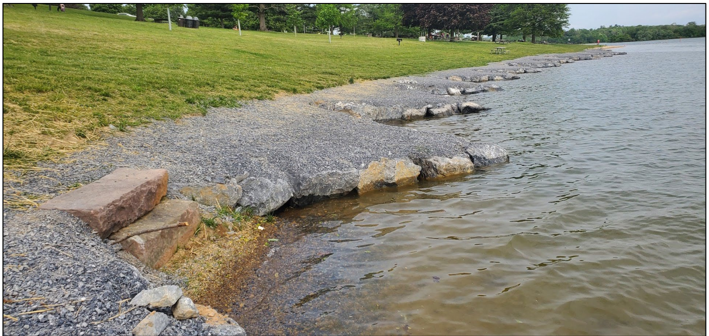
Figure 2: BCCD is part of a collaborative with the USACOE and PFBC. A 2022 NFHP Bass Pro Grant was awarded to the collaborative, and the grant funded assisted in the installation of rock framed deflectors along the shoreline. Flat stone was donated by the County to be utilized steps for water access for fishing, swimming, and boating. An education kiosk will be installed highlighting improvements and partnerships.
