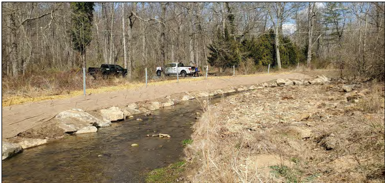
Figure 3: Native stone was used to create a rock toe along the stream channel. Soil lifts, erosion control matting, live stakes, and tree plantings were used to stabilize the streambank.
