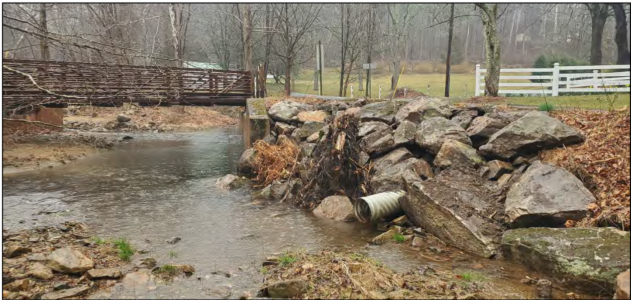
Figure 2: Native rock was imported from a local property and installed around 2 rootwads to deflect stormflows away from the bank and protect a foot bridge abutment.
