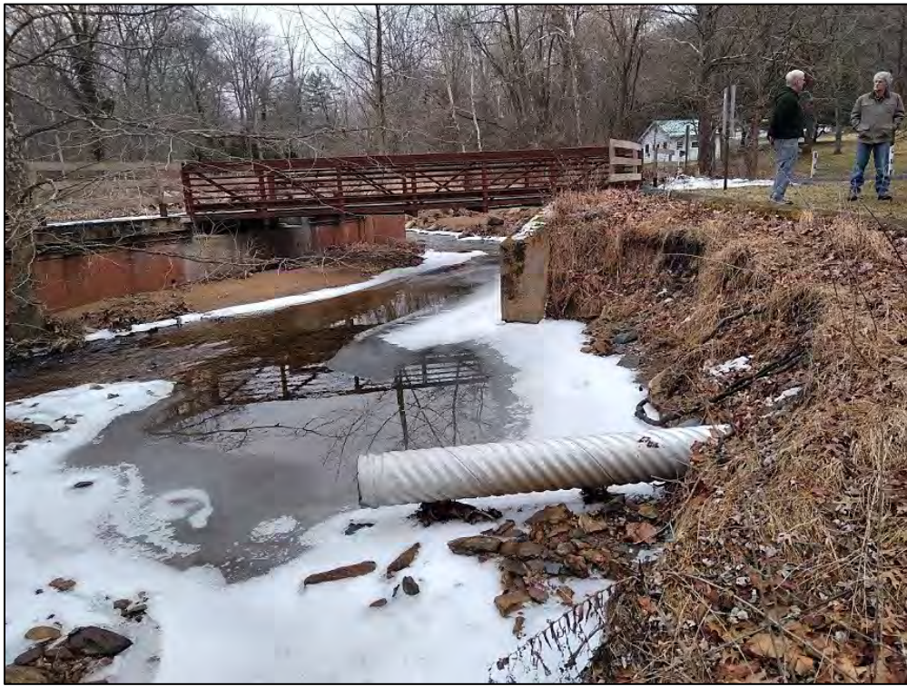
Figure 1: Back-to-back storms has scoured out ~ 8 ft. of streambank next to Township foot bridge abutment and Coult Property. Active erosion and significant downstream sedimentation is visible on Pine Creek an Exception Value stream in Pike Township, Berks County.
