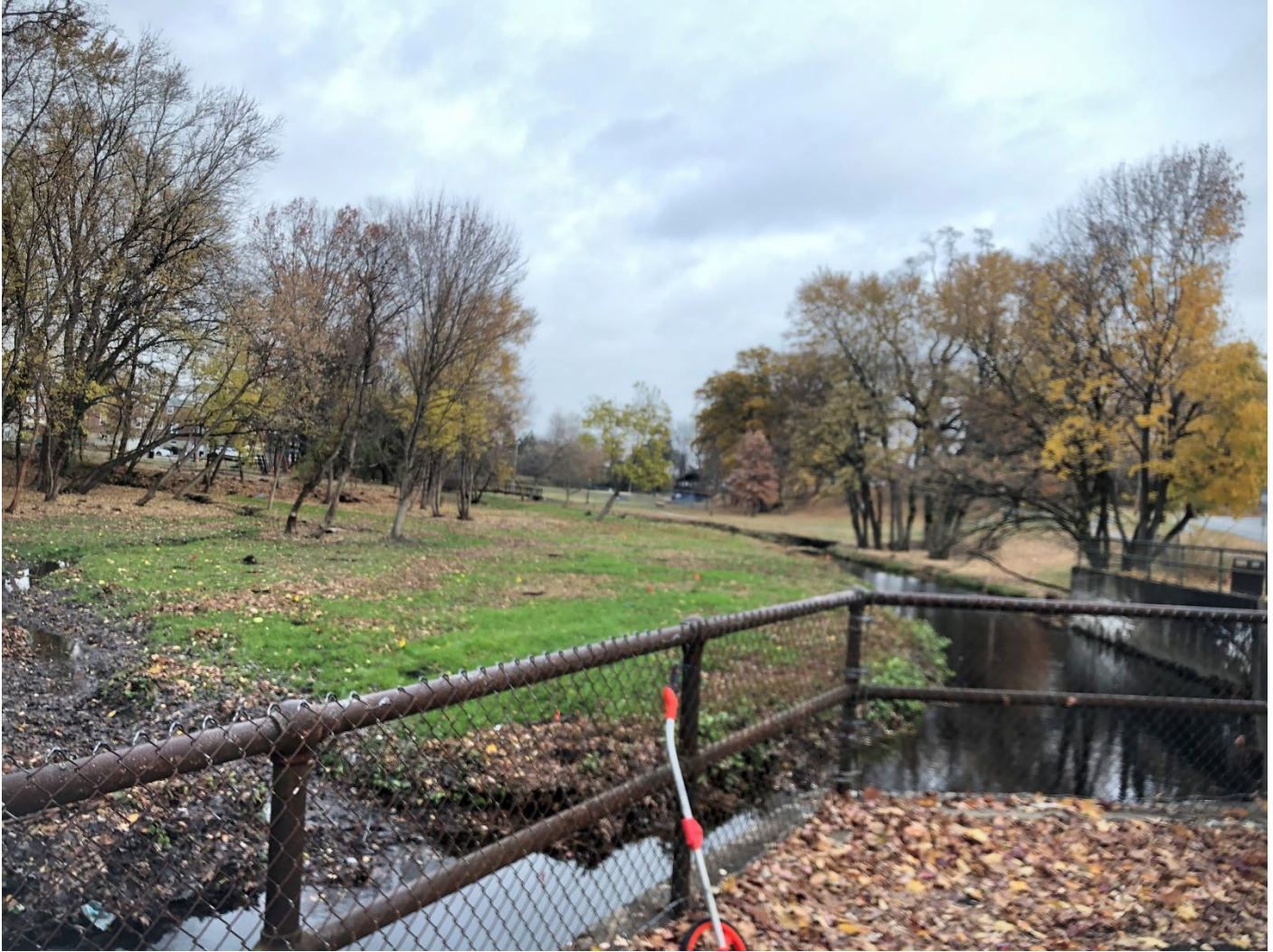
Figure 5 A look at one section of the project site prepared for plating after Invasive Japanese Knot Weed was mechanically controlled and grass was established to mitigate erosion. Note the holes are prepared by DCVA's Kyle Gaumann after the site had been flagged by DCCD's Watershed Specialist Chris Cook and Borough Concilman Paul K. Johnson (11/22/2024).
